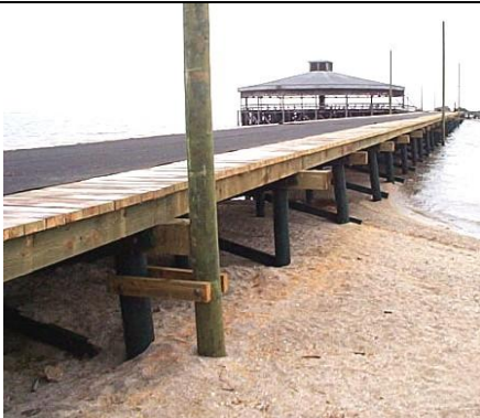
Coated Pilings & Posts
