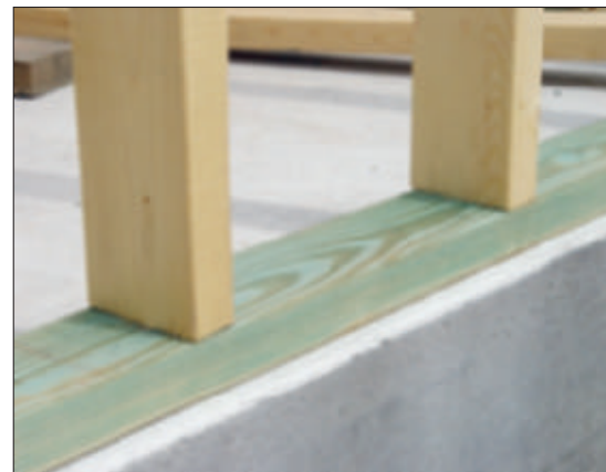
Building codes require that wood components in contact with concrete, masonry, or the ground be pressure treated or naturally durable.
